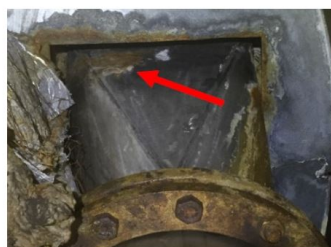
Cracks on water drain outlet (viewed from outside) with signs of leakage
