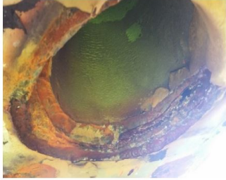
Cracks near distance piece leading to water ingress
