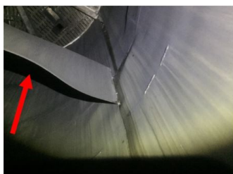
Deformed plates and buckled scrubber housing
