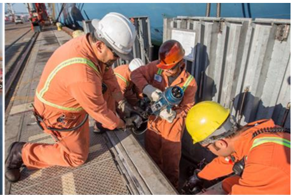
© Port of Los Angeles: Workers plug into the Port's shore power program
