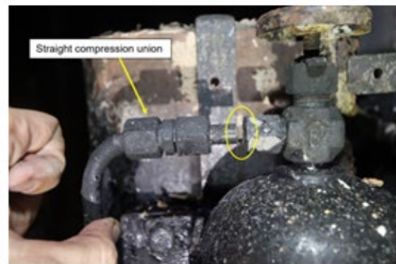
Fractured copper pipe
